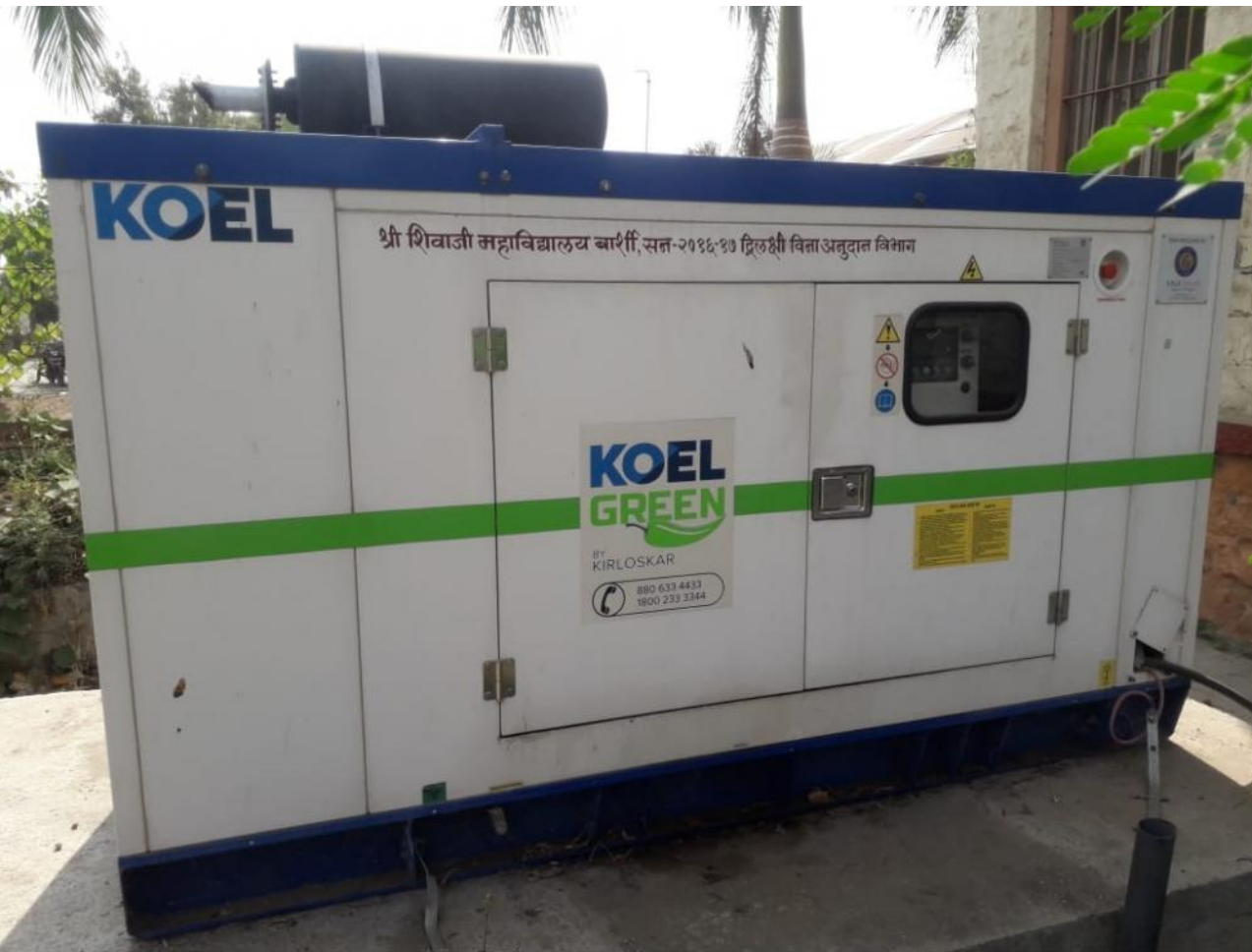
Generator of 30 KW capacity
