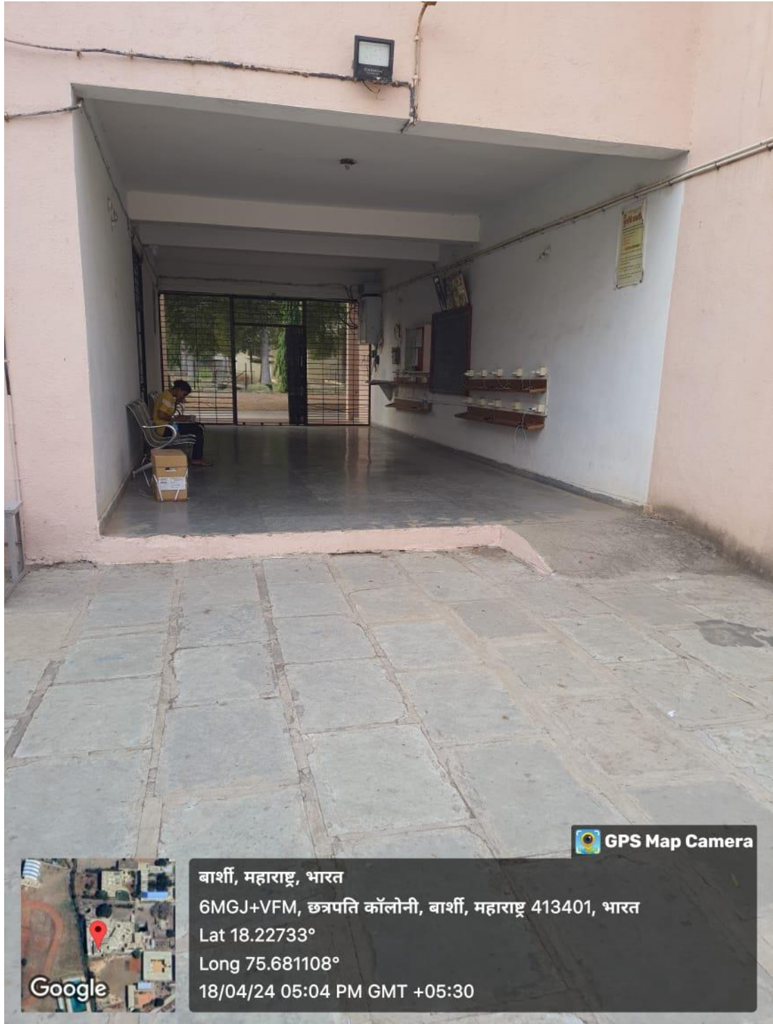
Mobile Charging Points for Students at Ladies Hostel
