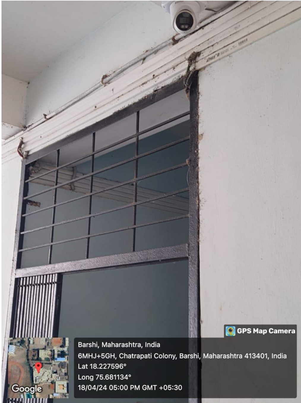
CCTV Cameras around Ladies Hostel
