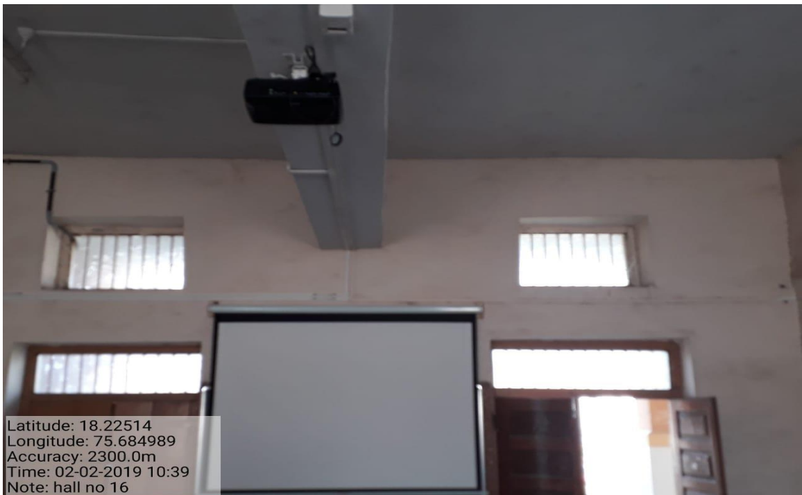
ICT Facility Hall No.16
