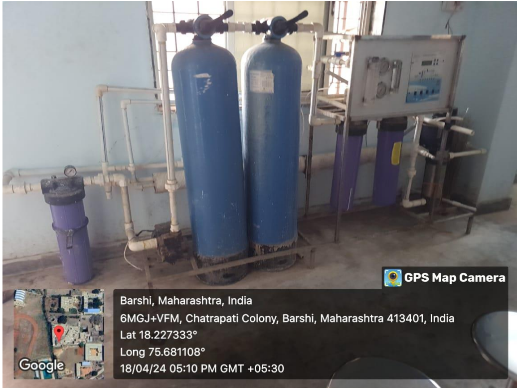
Water Filtration Unit in Ladies Hostel
