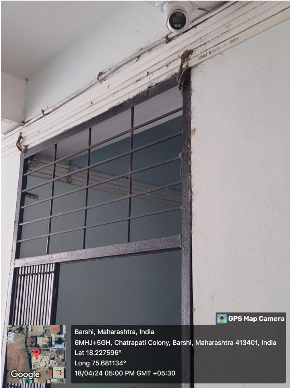
CCTV Cameras around Ladies Hostel
