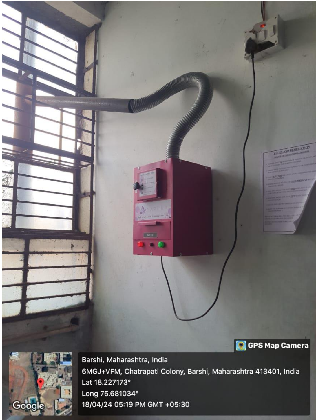
Disposable Machine for Sanitary Napkins on 1 st Floor of Ladies Hostel
