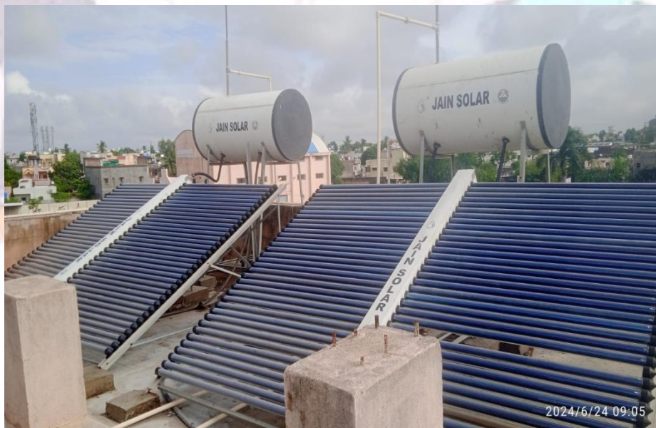
Solar Water Heater
